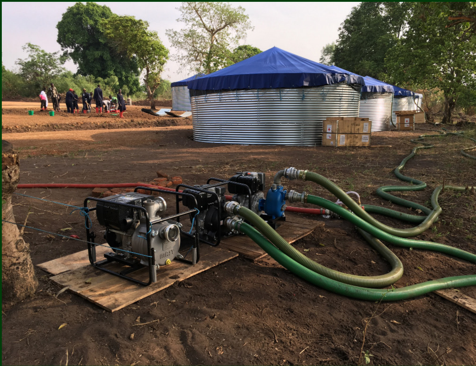
M40 Mass Sanitation Module Installation (Donated by Swedish Red Cross / Supplied by Butyl Products Group) Uganda, 2017
